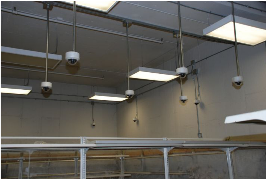
More than 80 cameras cover the facility including in the bullion vault.
